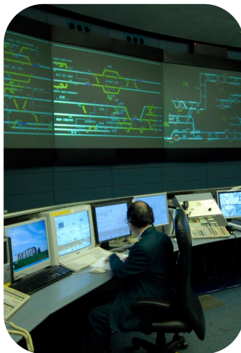
Railroad command signals
